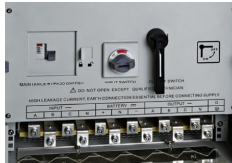
Manual bypass section of the 1.6 m cabinet.
